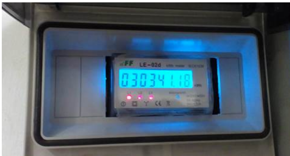
Smart meter from the monitored system. Source: Office of the capital city of Warsaw
